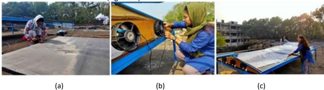
Figure 4. Different Parts of Dryer Construction (a) Preparation of tray, (b) Fan setting on Dryer, (c) set-up of plastic sheet
